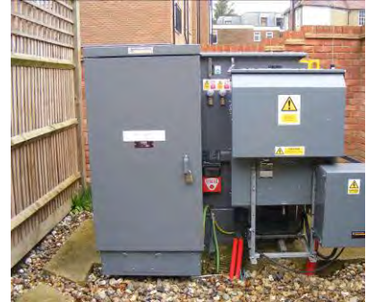
Figure 11 Newer design of compact ground-mounted substation
