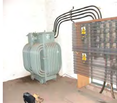
Figure 10 Older design of indoor substation
