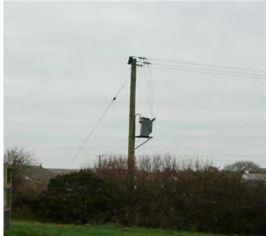
Figure 9 Pole mounted substation
